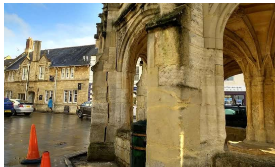
Photo 1.4.5d: Vehicle strike damage in 2018
