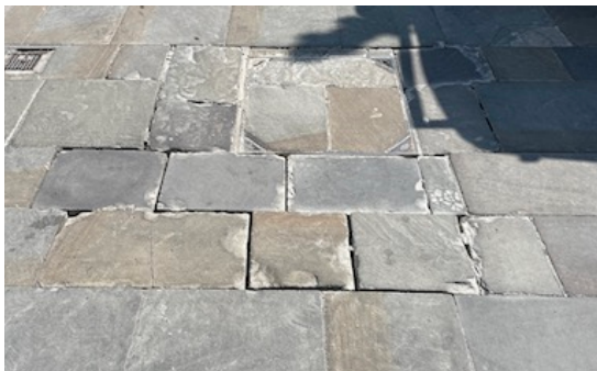
Photo 1.4.5c: Damaged paving from vehicles
